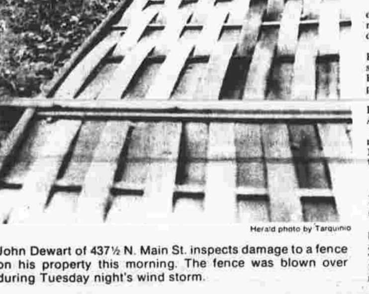
John Dewart of 437 1/2 N. Main St. inspects damage to a fence on his property this morning. The fence was blown over during Tuesday night's wind storm.
